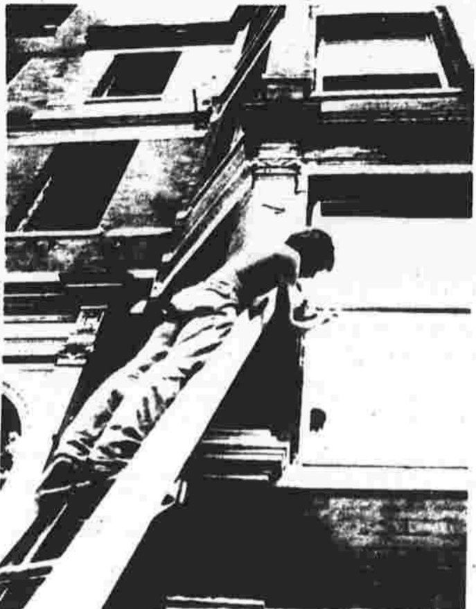
Worker repairs building soon to be turned into condominiums along Boston's Marlboro Street. College and university officials in Boston and across New England report the housing situation for their students is far from a sure thing due to the energy crunch, inflation, and condominium conversions. (UPI photo)
